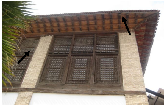
Figure2.17. Application of wood between roof and wall as well as between two floors in Kalbadiha's house, Sari, Mazandaran, Iran.
