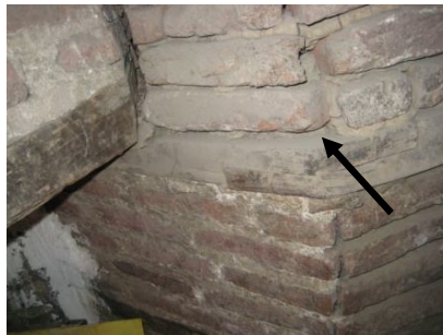
Figure2.8. Application of wood between the rows of bricks and the end part under the roof of staircase connecting to the roof area.
