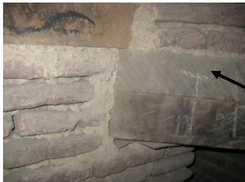
Figure2.9. Double wooden beams in the end part of staircase roof which are connected to the roof area.
