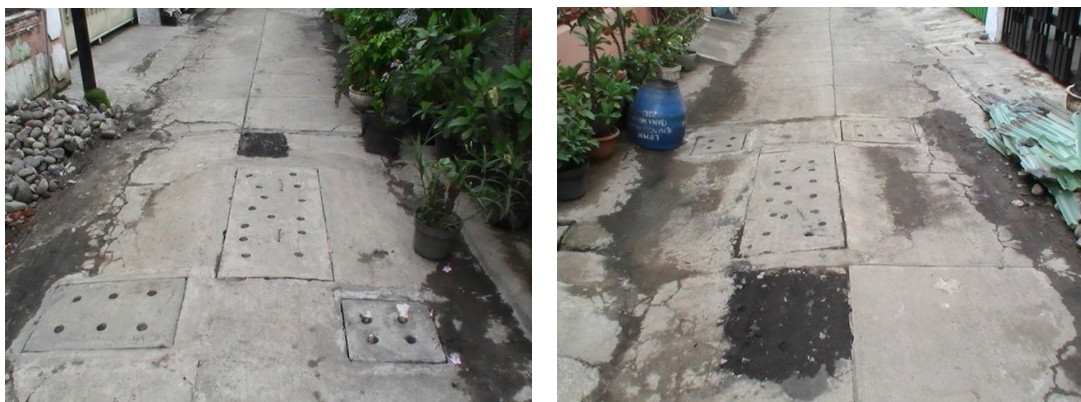
Figure 5 Ready Injection Well
